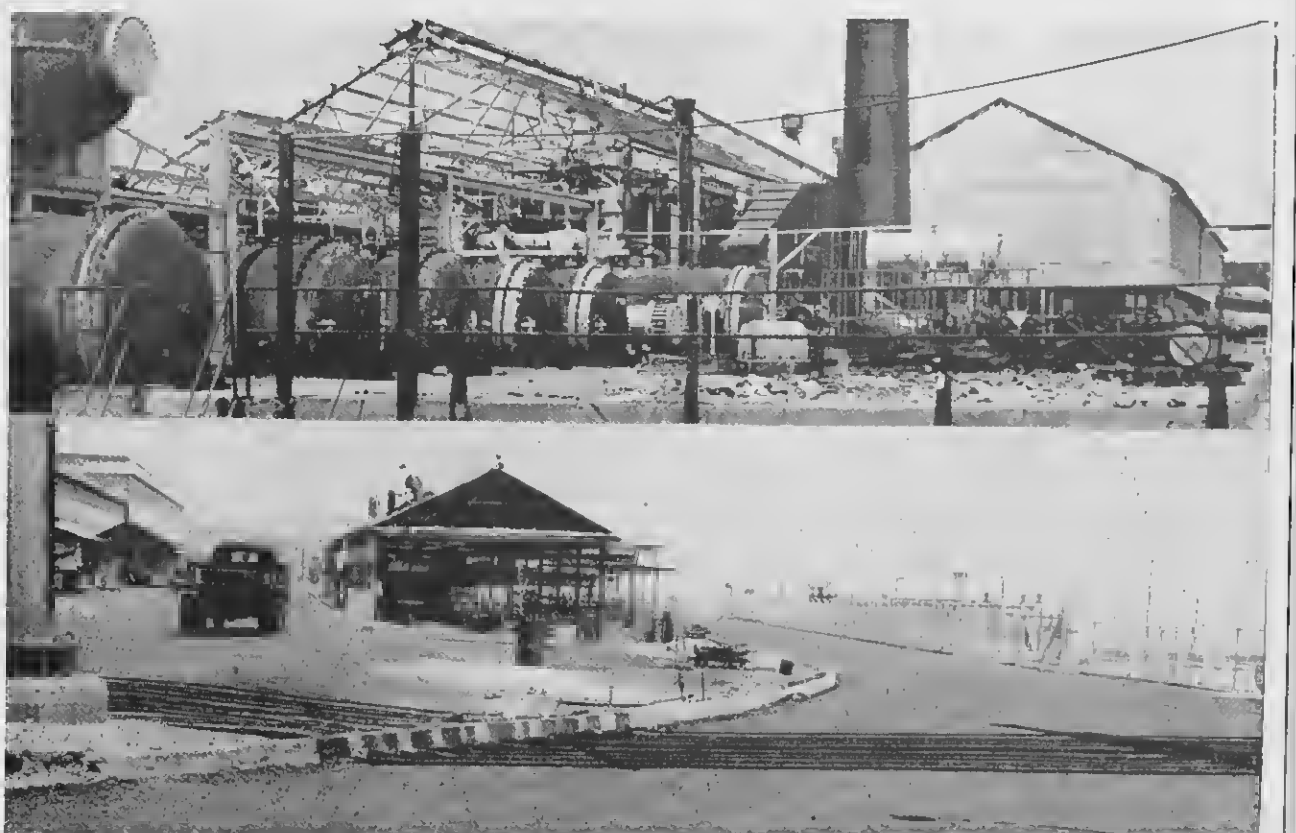
The old No. 3 evaporator plant is uprooted to make (Bottom picture) both the old road, left, and the new room for new storehouse space (top picture). This road, right, are shown. New section of shop will straddle space (16) will be warehouse space plus 600 sq. ft. of old road, while new road swings down past No. 1 & No. 2 Finger Piers.
